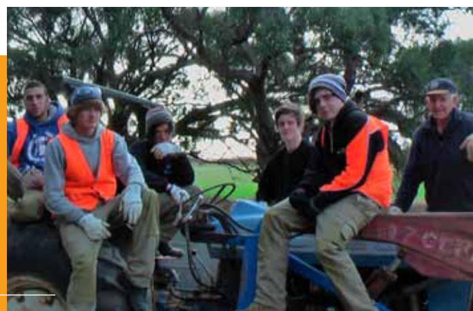
Left to right: Carpentry students Andrew Kasapidis, Dylan Walsh, Samuel Patton, Matthew Symons and Adam Withers helped Charlton farmers rebuild damaged fences.
